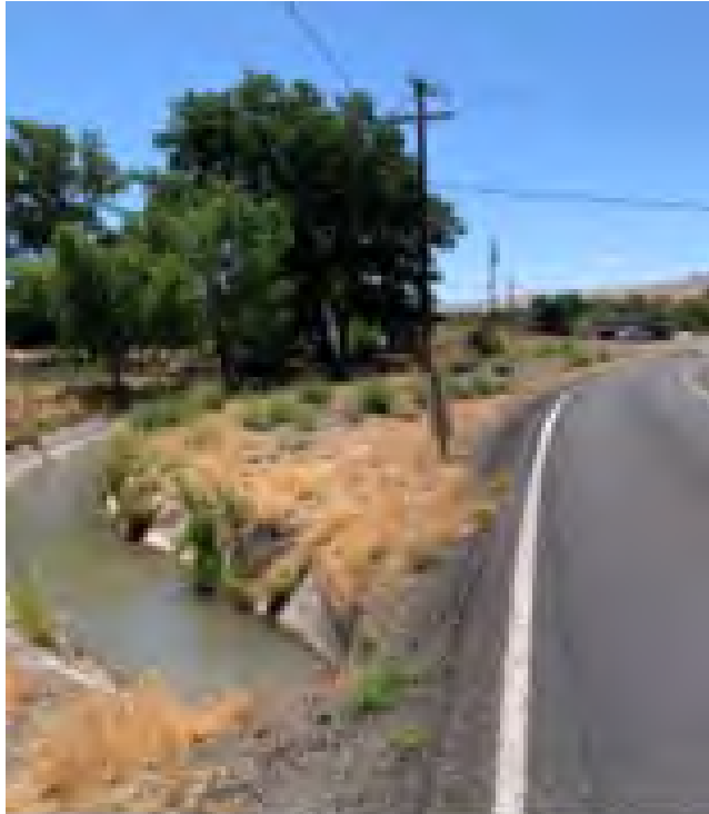
Picture 3: Unprotected Culvert the east side of Route 447 (looking south)
